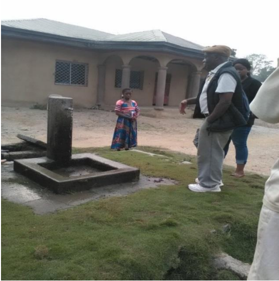
Poorly maintained stand tap
