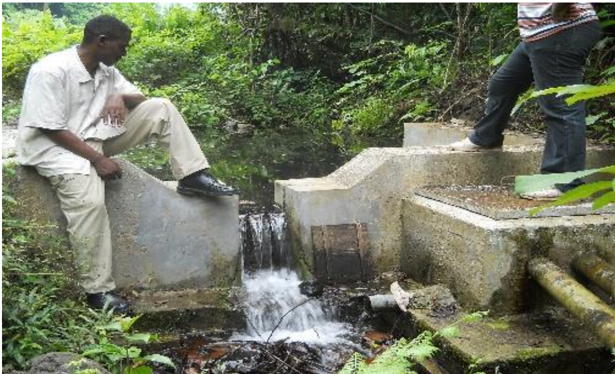
Intake of a steam water source
